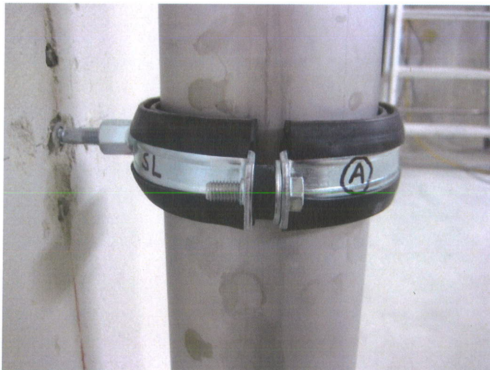
Figure 5 Wastewater installation system "ACO pipe" consisting of stainless steel pipes and fittings (manufacturer: ACO Industries k.s.) mounted with acoustic pipe clamps "Bismat 1000, one spacer" (manufacturer: Walraven). The guidance clamp (SL) and the sliding clamp (SL) were mounted with 7 mm space between the locking tabs of the clamp (one spacer on each side). Upper picture: "ACO PIPE" with double clamp "Bismat SL and Bismat SX" in the upper wall area. Lower picture: "ACO PIPE" with sliding clamp "Bismat SL" in the lower wall area
